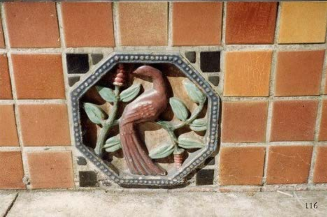
116. 16 th St. & Guerrero, S.F. (S&S vent tile set in mortar; all remaining tilework painted black)
