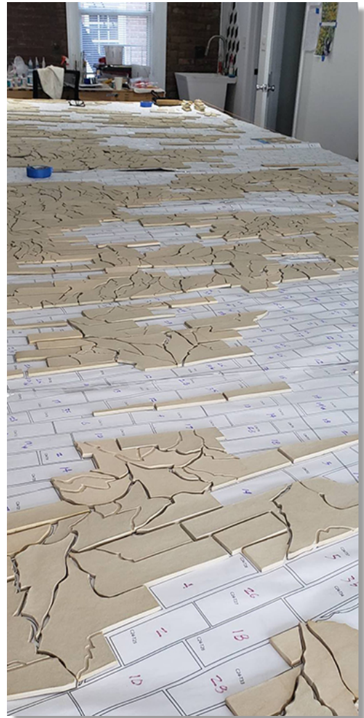
Bisque-fired pieces are placed on each of three 7' x 21' design templates. Note that the grout joints between pieces are created by the shrinkage of the clay during the firing.
